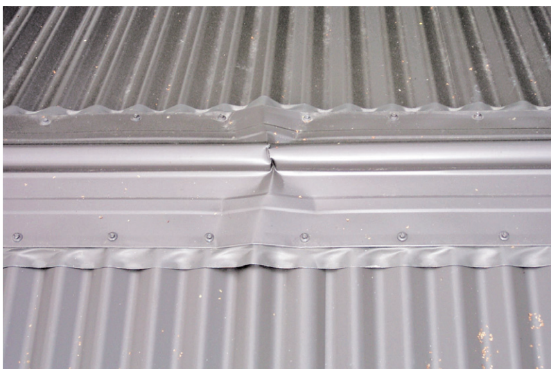
Figure 2 Buckled change of pitch flashing
